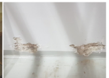
Damaged wall by forklifts
