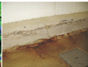
Damaged concrete kerb
