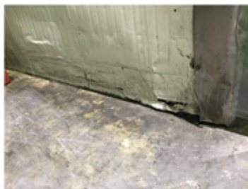
Damaged sandwich panel
